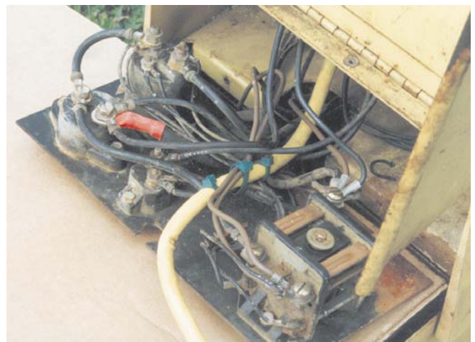
Below: The opened access panel on an E10. The larger relay on the right is the PTO contactor.
